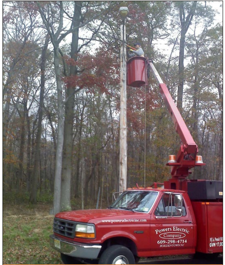
Workers repair lights outside the LSB lobby, where an electric line to streetlights was damaged.
