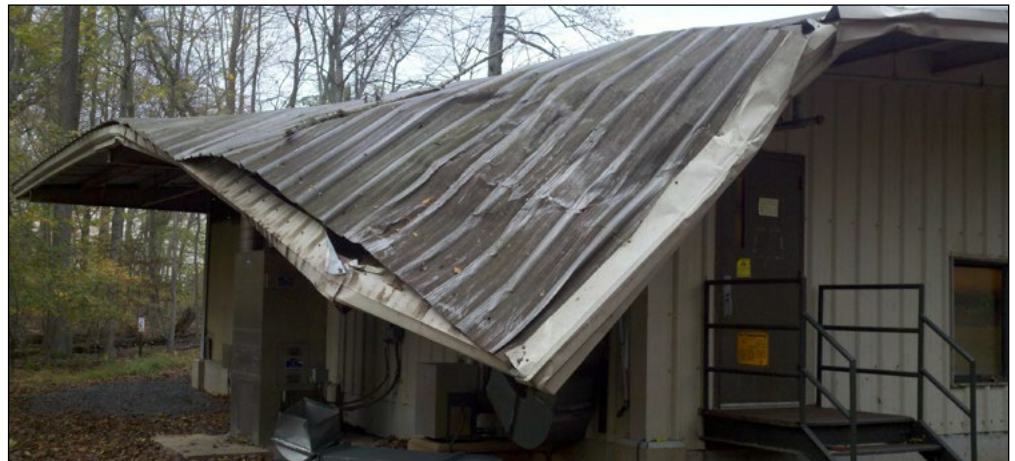
A tree damaged an awning at the Haz Mat Building.
