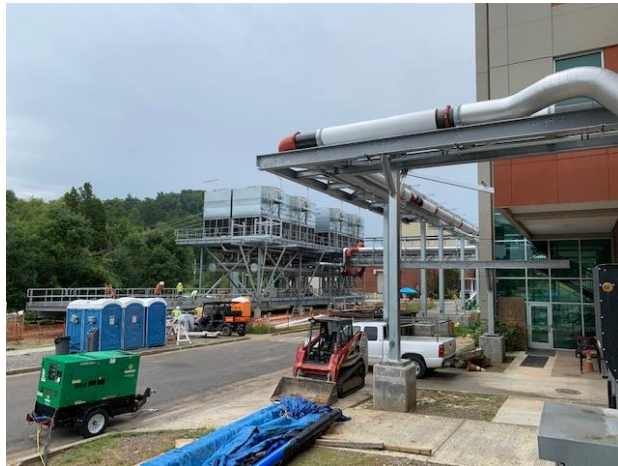
Piping with cooling towers
