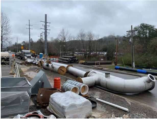
Cooling Water Pipes
