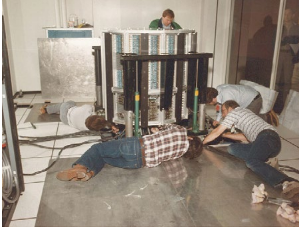
Staff at the National Magnetic Fusion Energy Computer Center install a Cray-2 machine.
