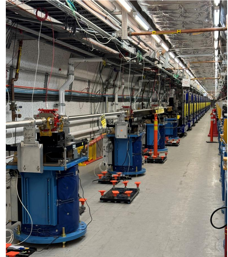
Space upstream of the existing Soft X-Ray (SXR) Undulator is prepared in August 2024 for the addition of nine LCLS-II-HE units.
