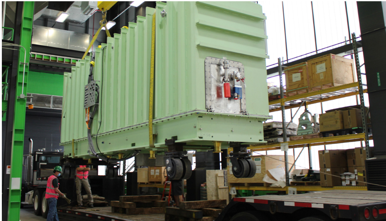
Fig. 3.2. Facility Construction Continues During the Pandemic. Workers at the Facility for Rare Isotope Beams (FRIB) at Michigan State University move a cryomodule into the linear accelerator (linac) tunnel. As the start of user operations in early 2022 nears, the FRIB team commissioned the entire linac, including all 46 cryomodules, in April 2021. The commissioning team was distributed to five separate control rooms to comply with COVID-19 workplace safeguards. [Courtesy Michigan State University]
