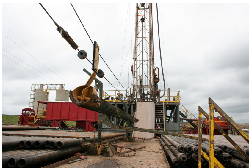
Figure 5-2 Typical drilling operations of a CO 2 injection well. Source: R. A. Esposito, Southern Company.
