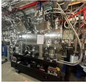
Nb 3 Sn SCU on the APS storage ring
