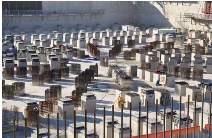
The Tokamak Pit
