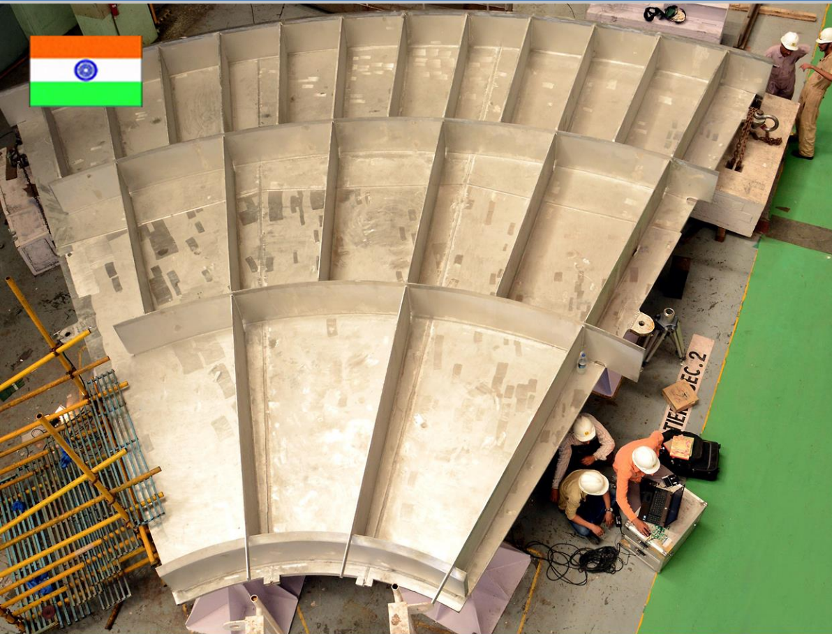
Cryostat base fabrication at Larsen & Toubro in Hazira, India (December 2014). Photo: ITER India
