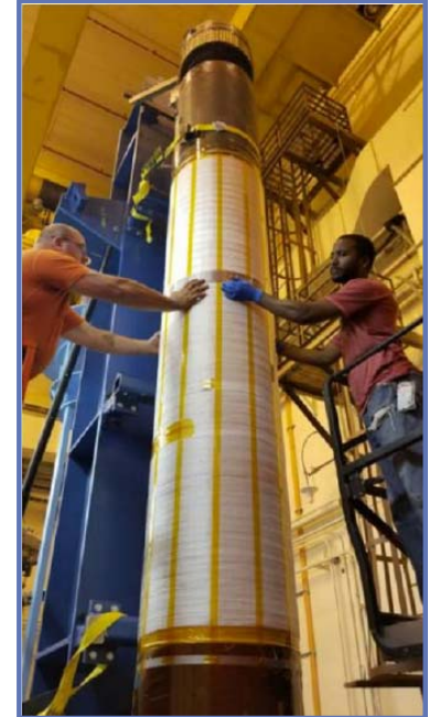
TF/OH conductor bundle prior to a casing fit-up lift
