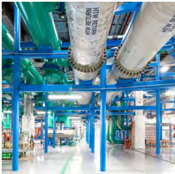
Fig. 3.9. The newly built central energy plant serves power and cooling to the high-performance computing systems of the Oak Ridge Leadership Computing Facility, including the soon-to-be launched Frontier supercomputer. [Courtesy Oak Ridge National Laboratory]
