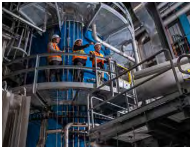
Fig. 3.7. A view inside the Facility for Rare Isotope Beams (FRIB) cryogenic plant. The vertical cold box (in blue) works together with the horizontal cold box to cool helium to 4.5 K. FRIB's beam-accelerating cryomodules contain superconducting radio frequency resonators that must operate at temperatures a few degrees above zero to be superconducting. The 4.5 K liquid helium makes the resonators superconducting. [Courtesy Facility for Rare Isotope Beams]
