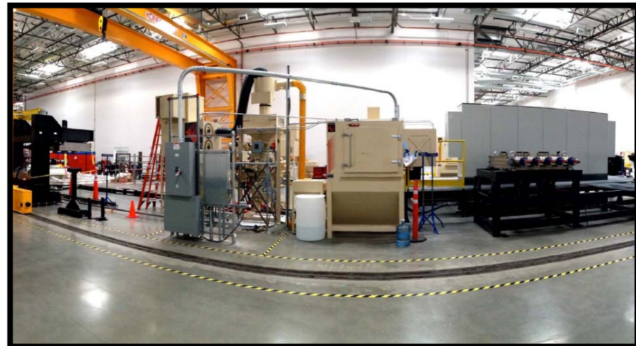
Installation of the first winding station for the central solenoid at General Atomics (San Diego, CA)
