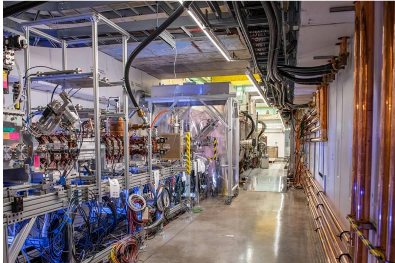
PIP II Integration Test Facility (PIP2IT)
