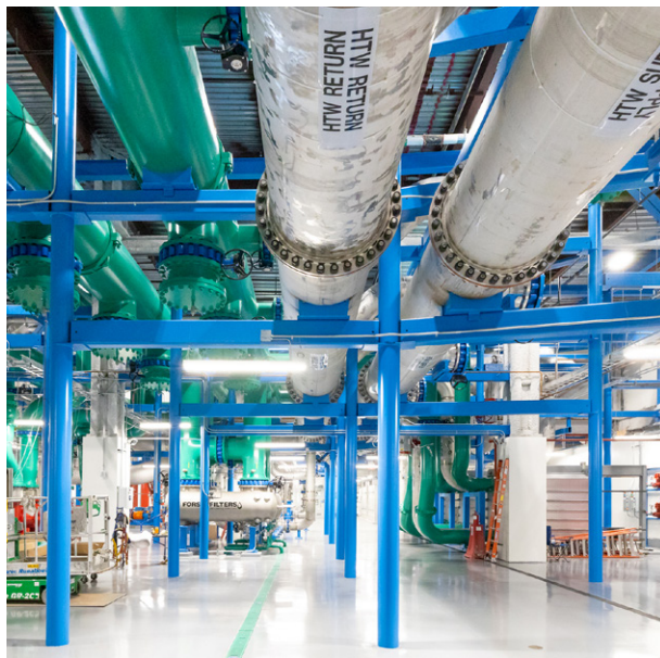
Fig. 3.9. The newly built central energy plant serves power and cooling to the high-performance computing systems of the Oak Ridge Leadership Computing Facility, including the soon-to-be launched Frontier supercomputer. [Courtesy Oak Ridge National Laboratory]
