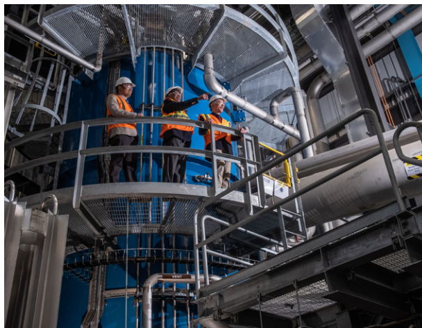
Fig. 3.7. A view inside the Facility for Rare Isotope Beams (FRIB) cryogenic plant. The vertical cold box (in blue) works together with the horizontal cold box to cool helium to 4.5 K. FRIB's beam-accelerating cryomodules contain superconducting radio frequency resonators that must operate at temperatures a few degrees above zero to be superconducting. The 4.5 K liquid helium makes the resonators superconducting. [Courtesy Facility for Rare Isotope Beams]
