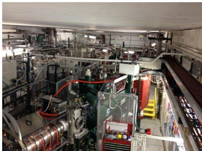
Stopped beam facility (N4 vault)
