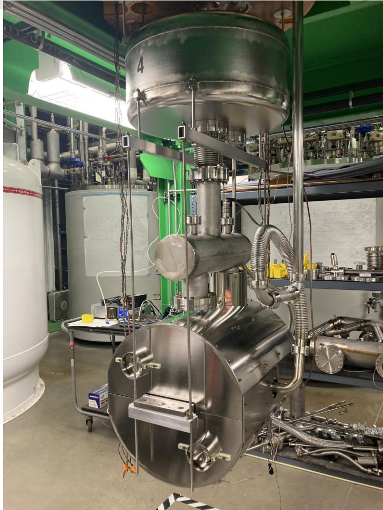
MGS installed on the SC53-159.
