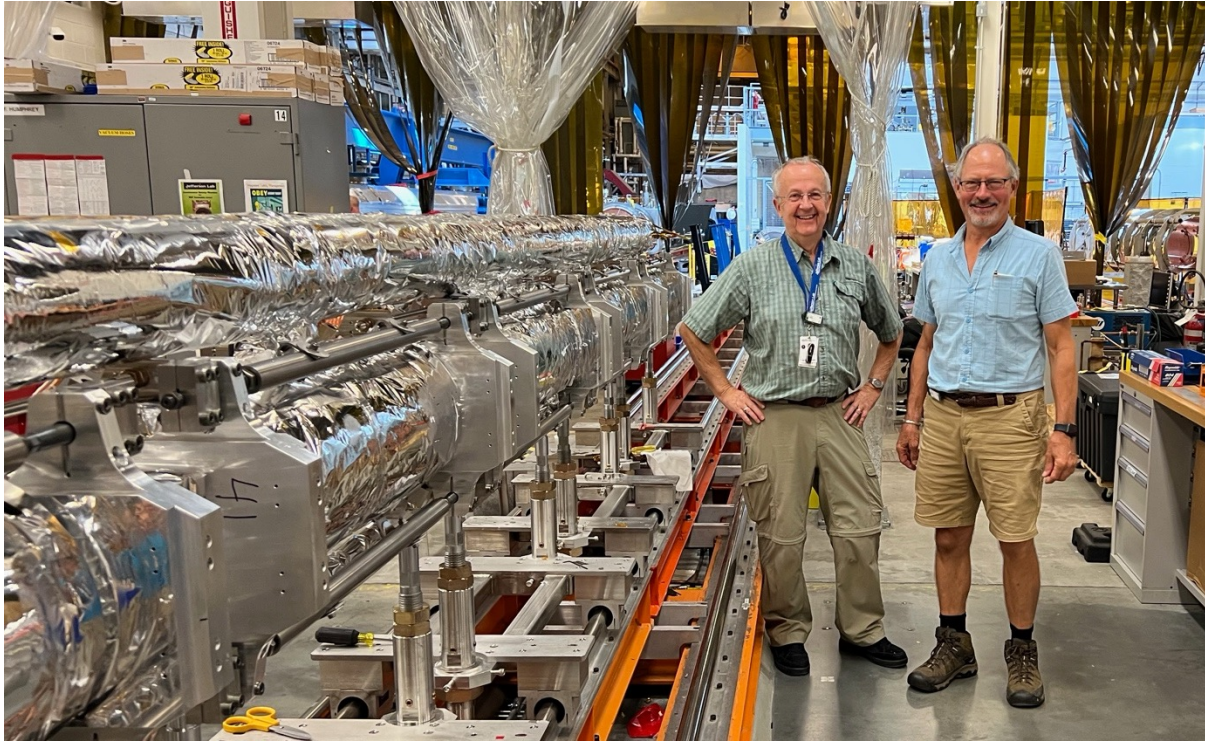
George Biallas and Kevin Jordan setting up for installation in full C100 cryomodule
