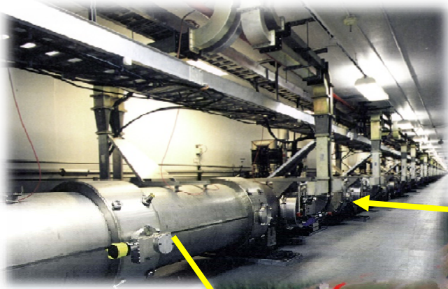
Cryomodules in the accelerator tunnel
