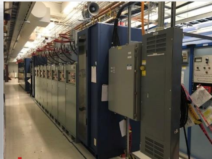
LCLS II Equipment Racks
