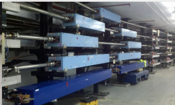
~500 Large Dipoles powered by >40 HVPS
