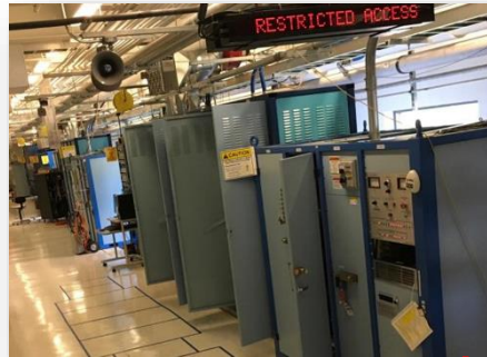
LERF Equipment Racks
