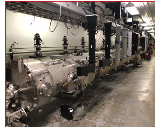
Refurbished C100 installed
