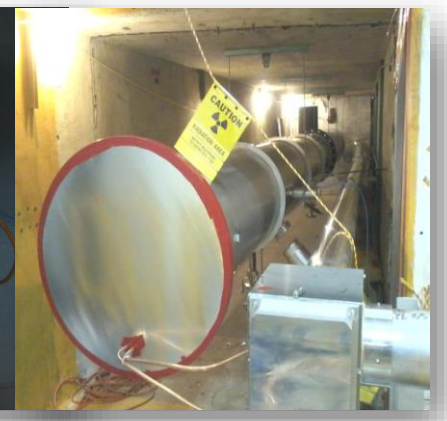
High Power Exp Hall Beam Dump
