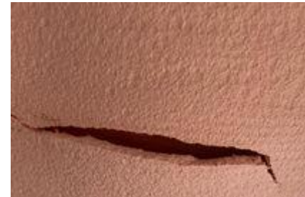
Cold sprayed Cu layer cracked
