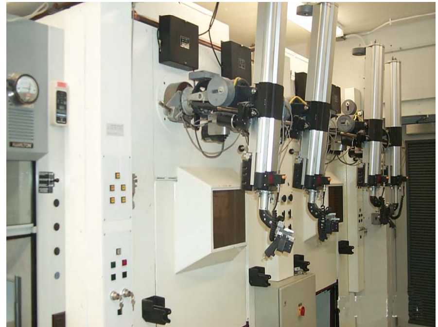
View of several processing hot cells
