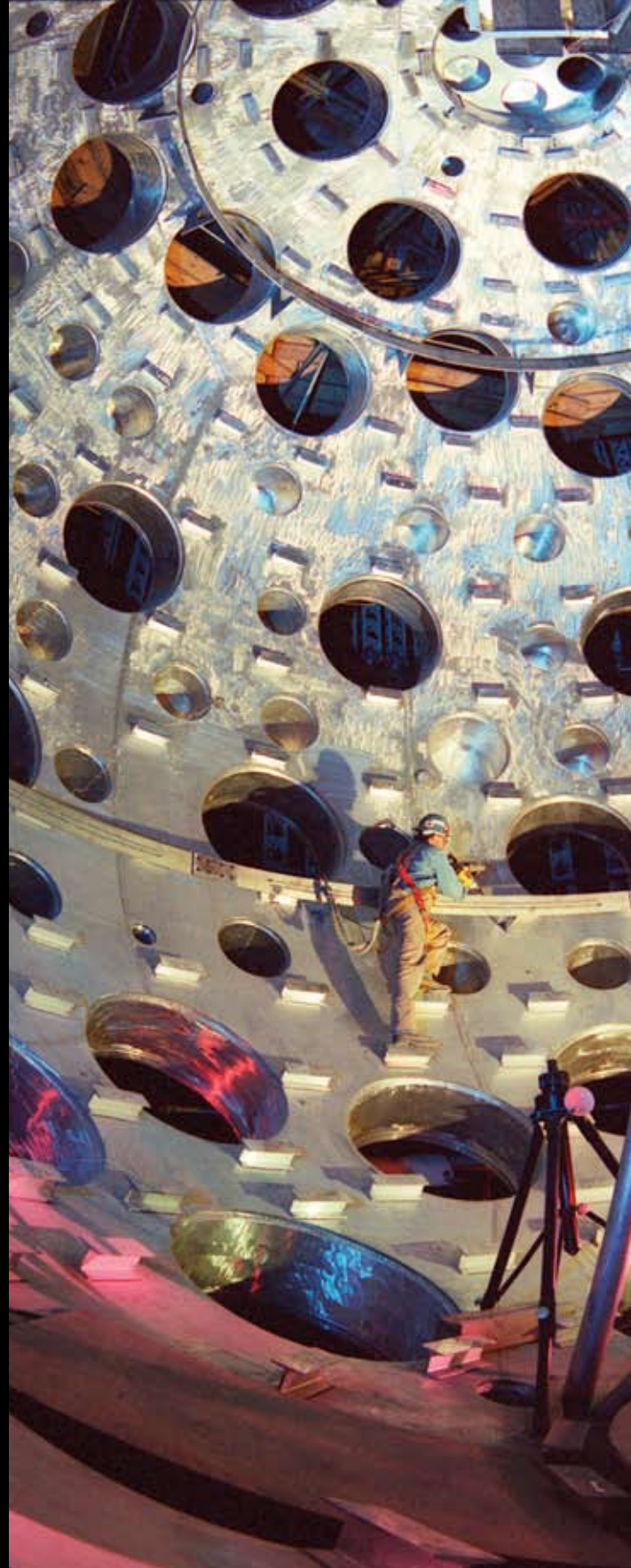
Construction workers install equipment inside the 10-meter diameter target chamber at the National Ignition Facility. The chamber, a sphere 10 meters in diameter, was assembled from ten-centimeter-thick aluminum panels which were preformed and then welded in place. It is covered with 0.3 meters of concrete which has been injected with boron to absorb neutrons from the fusion reaction. The target chamber is filled with holes that are needed to permit the laser beams to enter the chamber and to provide viewing ports for all of the diagnostics.
