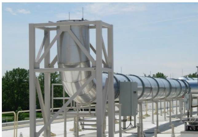
3410 Building Filtered Exhaust Stack
