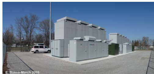
Sodium Sulfur Battery 2 MW
